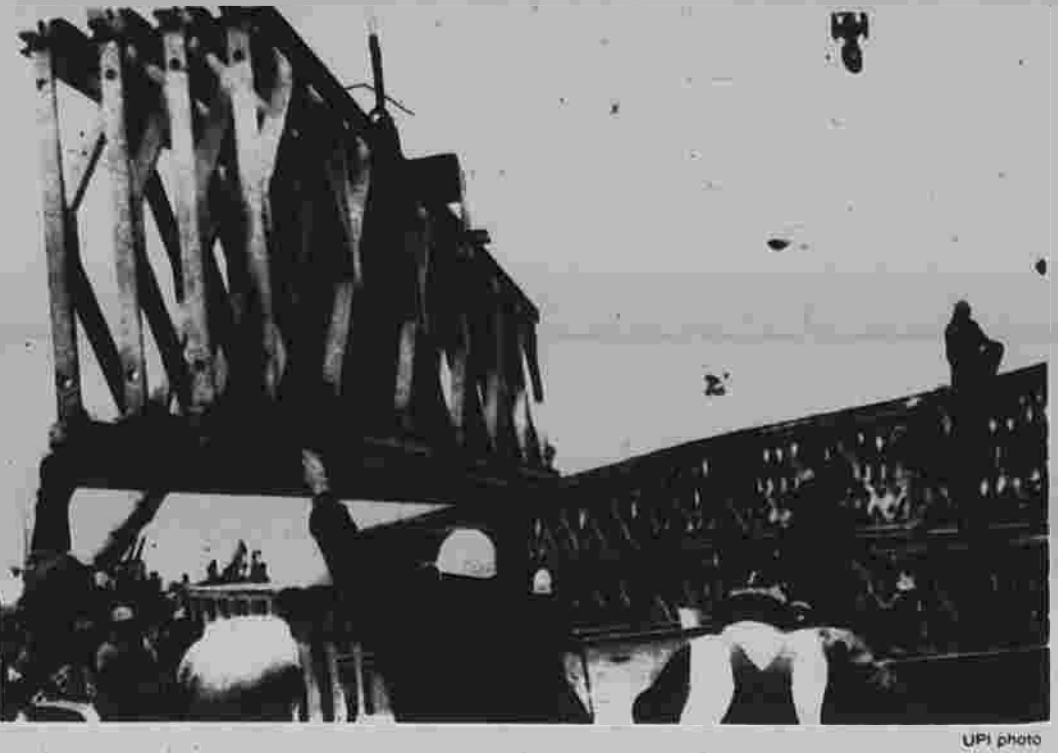
Workers dismantle the temporary span over the Mianus River on the Connecticut Turnpike at Greenwich Thursday. Southbound lanes will carry two-way traffic until the permanent bridge is completed. A section of the Mianus bridge collapsed June 28, 1983, killing three people.
